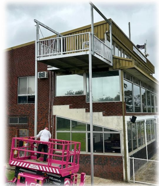
Joe Paterniti moving the scissor lift into place for install of the west face steel
