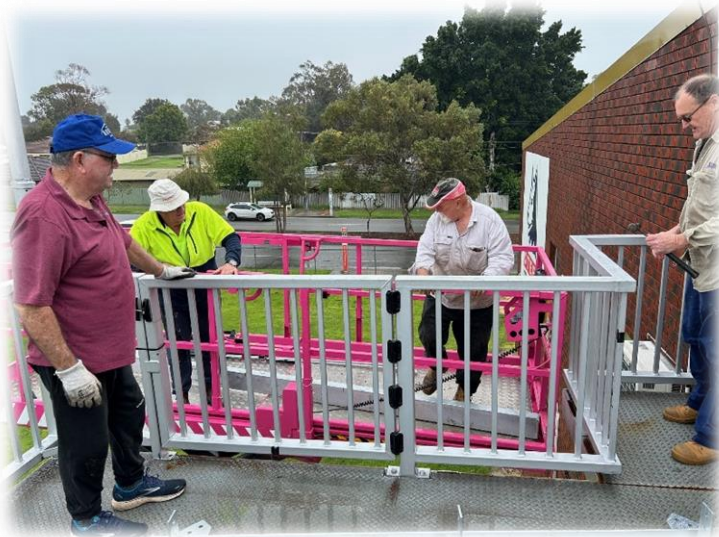
All hands-on deck ready to install the first column. From left, Rod Greene, Gary Cox, Joe Paterniti and Trevor Hoy (photo by Ross Wheldon)
