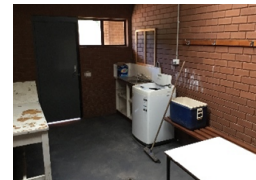
Poor condition (multiple quality issues)
