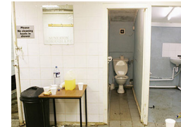
Very poor condition
