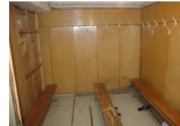
Poor condition (multiple quality issues)
